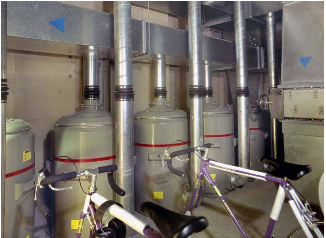
Filter units in the AC plant room. These were installed during the 1989 upgrade. Photo Nick Catford
